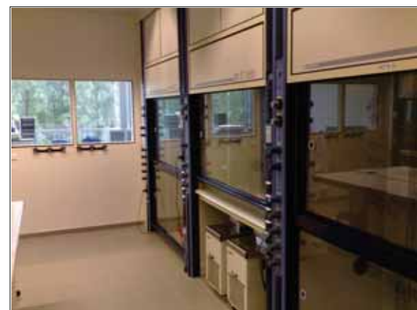
CMR Fume Hood Controllers in operation
